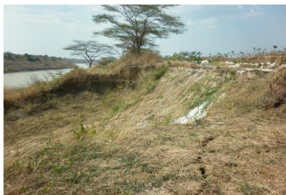
Gambar 4 Longsoran tebing sungai
